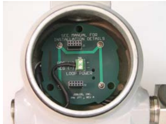
Photograph No. 2 Termination Board
